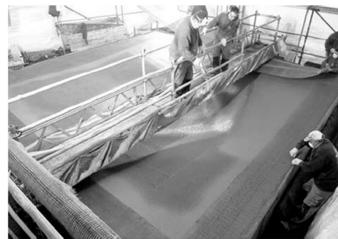
Figure 13: Manufacturing of the TRC hyper-shell layer by layer by shotcrete [photo: © RWTH Aachen], [38]
