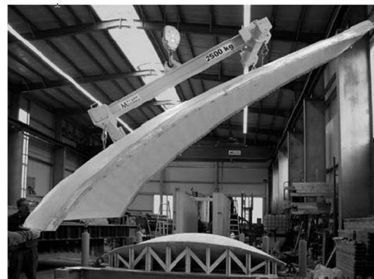
Figure 10: Demolding of a hardened shell element in the concrete yard in Kahla/Saxony [photo: Daniel Ehlig, TU Dresden]
